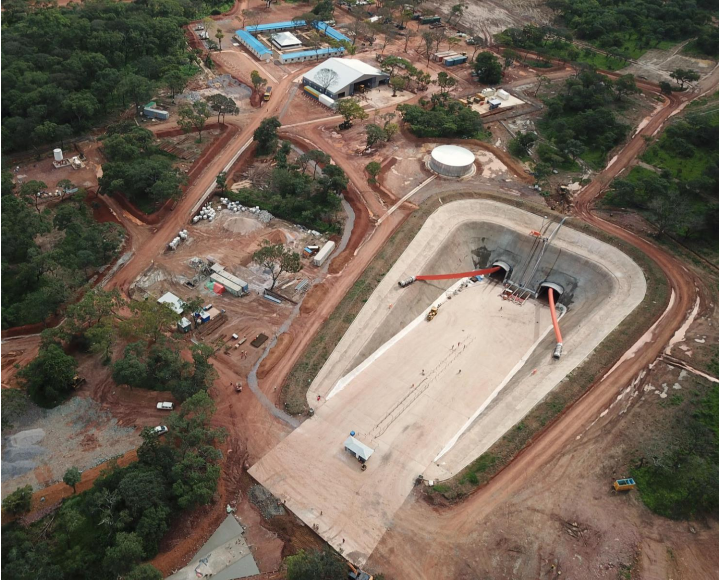
Aerial view of the Kakula box cut, showing portals for the twin declines, and related surface facilities.
