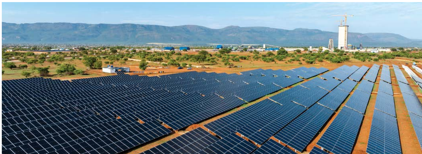
A close-up view of Platreef's on-site 5MW Solar PV plant with Shaft #2 visible in the background.
