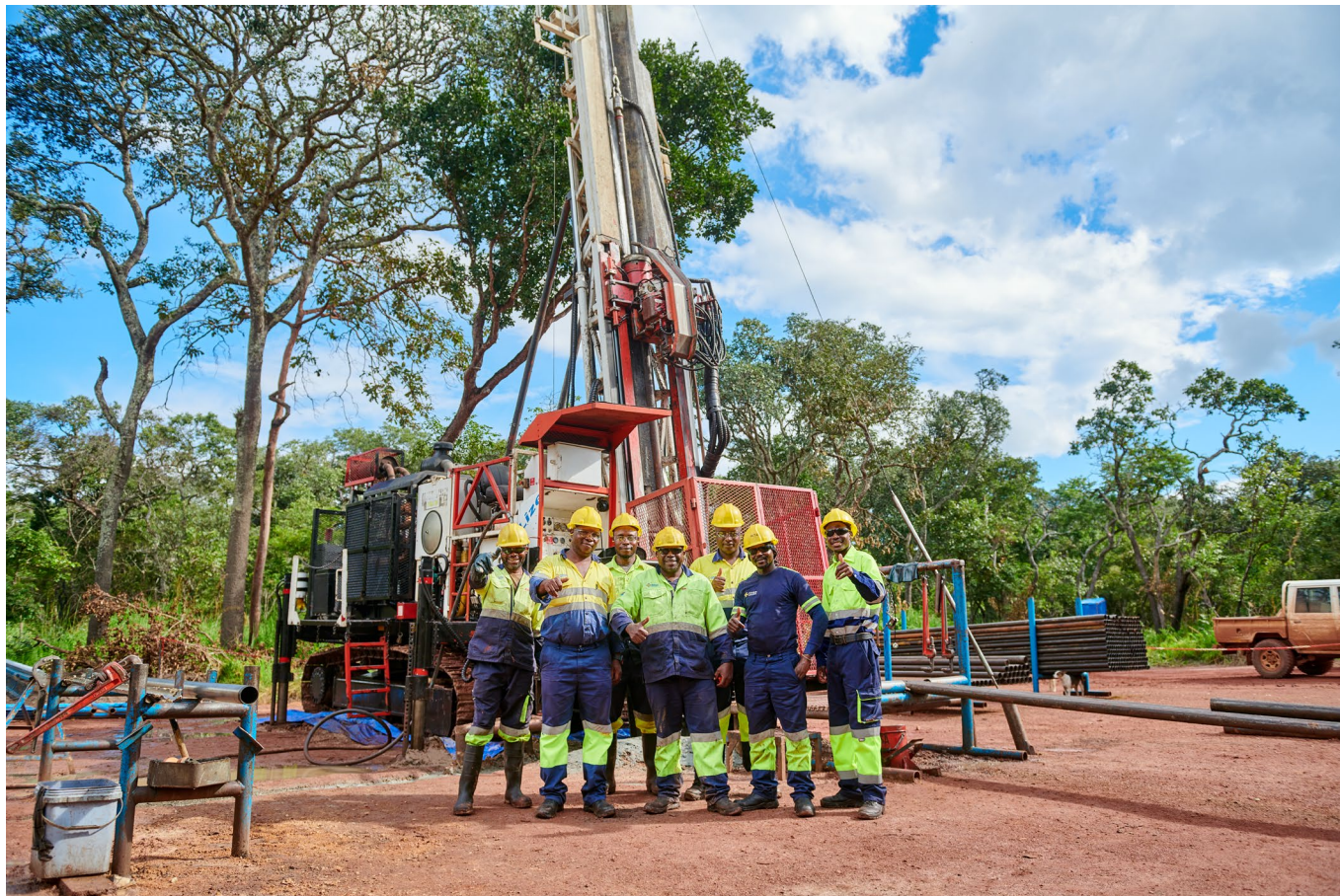
Photo: A diamond drilling crew from Titan Drilling of Lubumbashi, DRC, drilling in the Western Forelands
