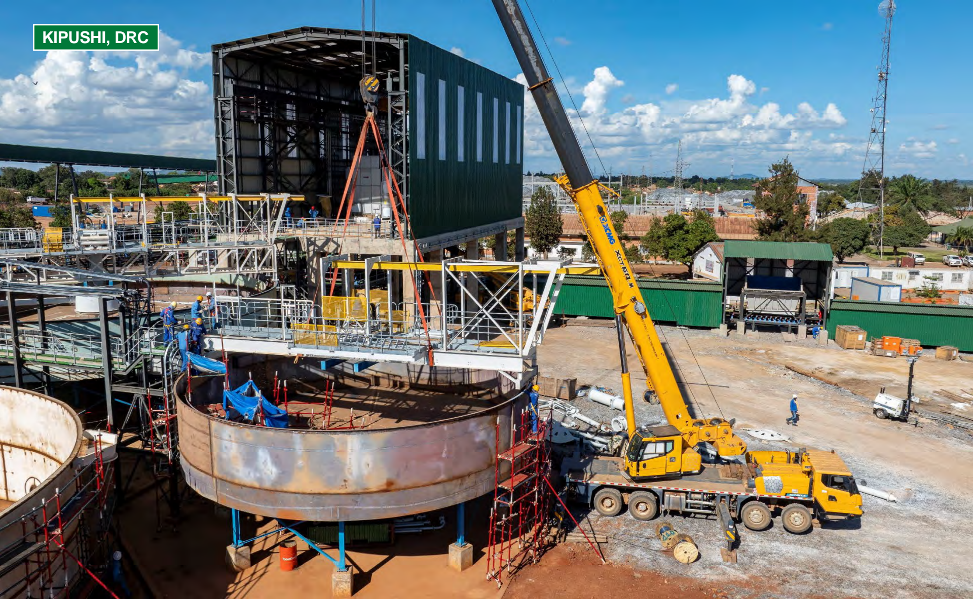
Mechanical equipment installation progress at Kipushi's process plant. Kipushi is ahead of schedule for first production in Q2 2024.
