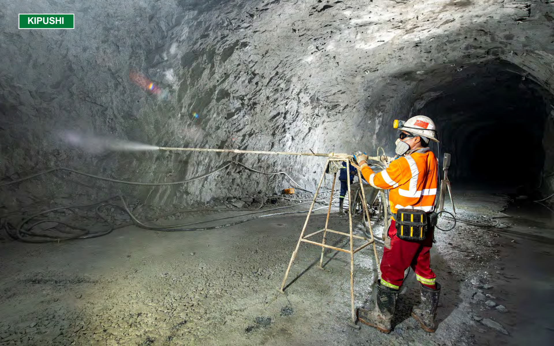
Richard Kayembe applying thin spray liner in one of the drill drives underground at the 1320-metre level.
