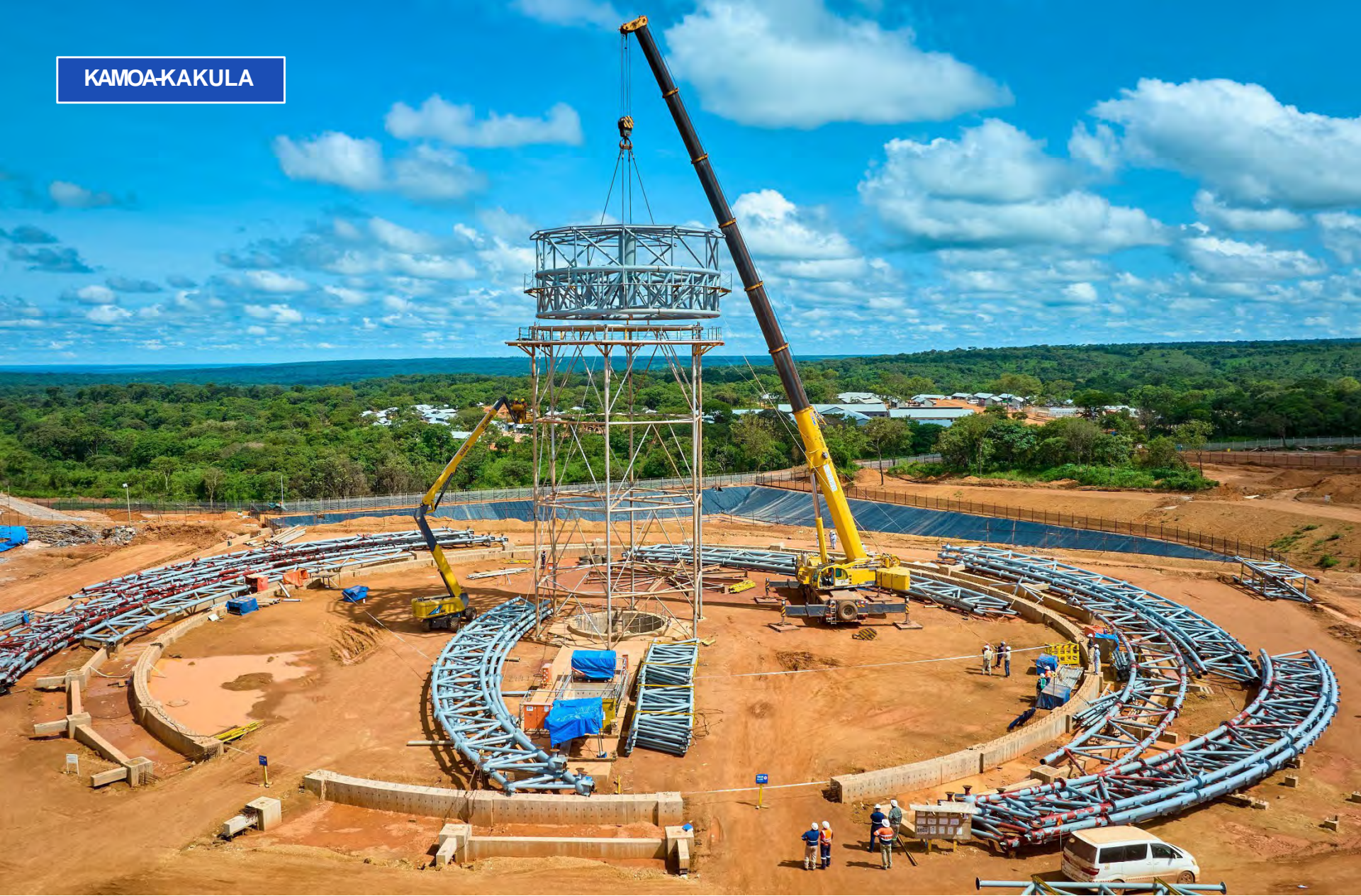
Cranes lift the central ring of the smelter's concentrate-blending building into place.
