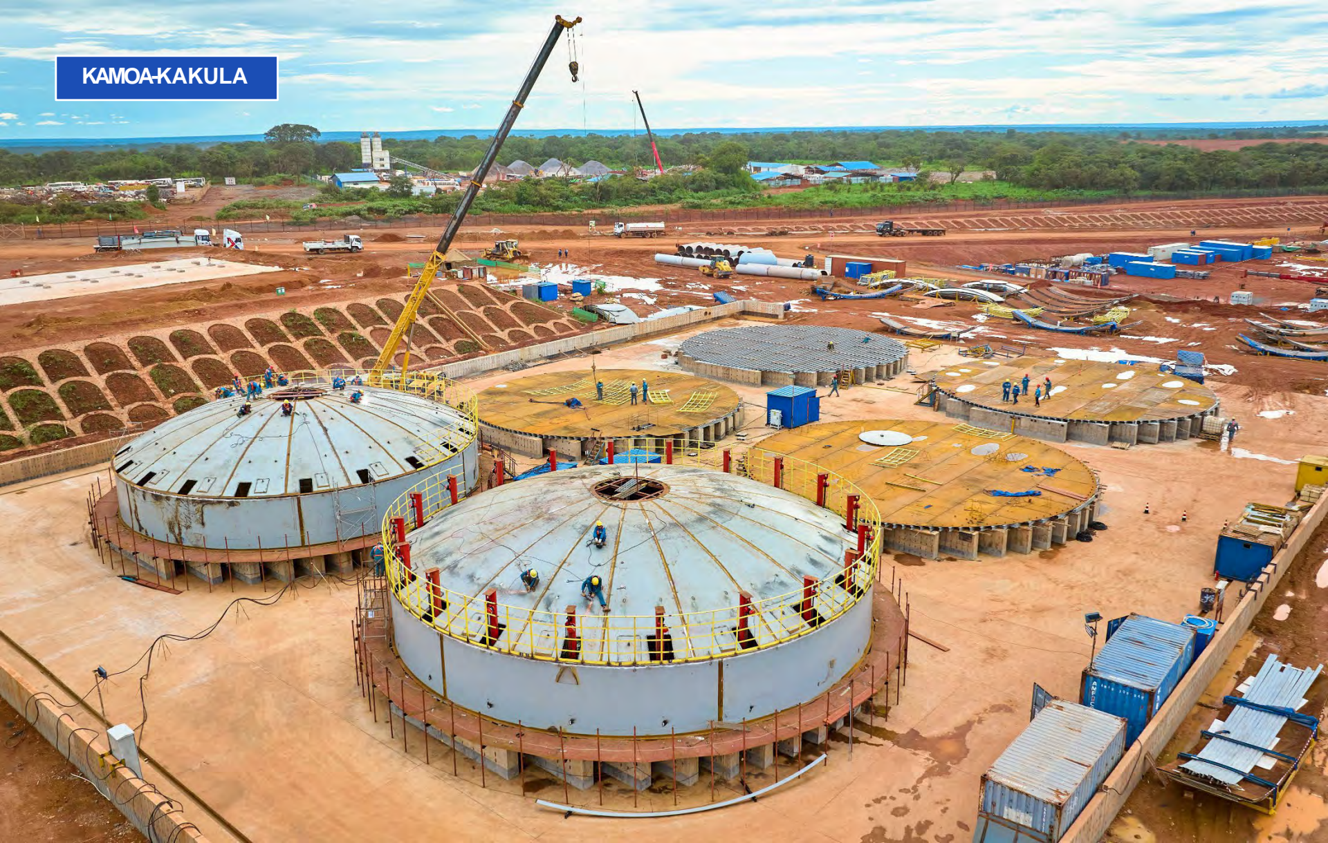
Assembly progresses on the high-strength acid storage tanks at Kamoa-Kakula's smelter project.
