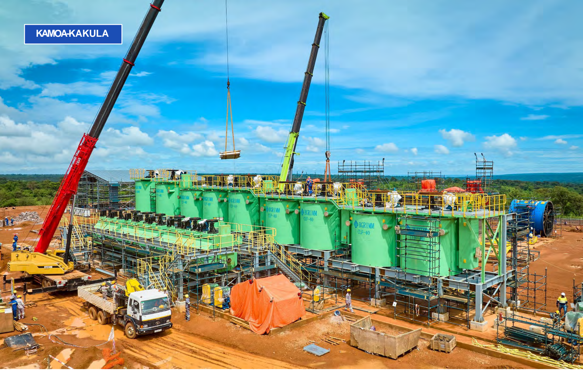
Construction cranes and crew members at work on the smelter's slag flotation cells.
