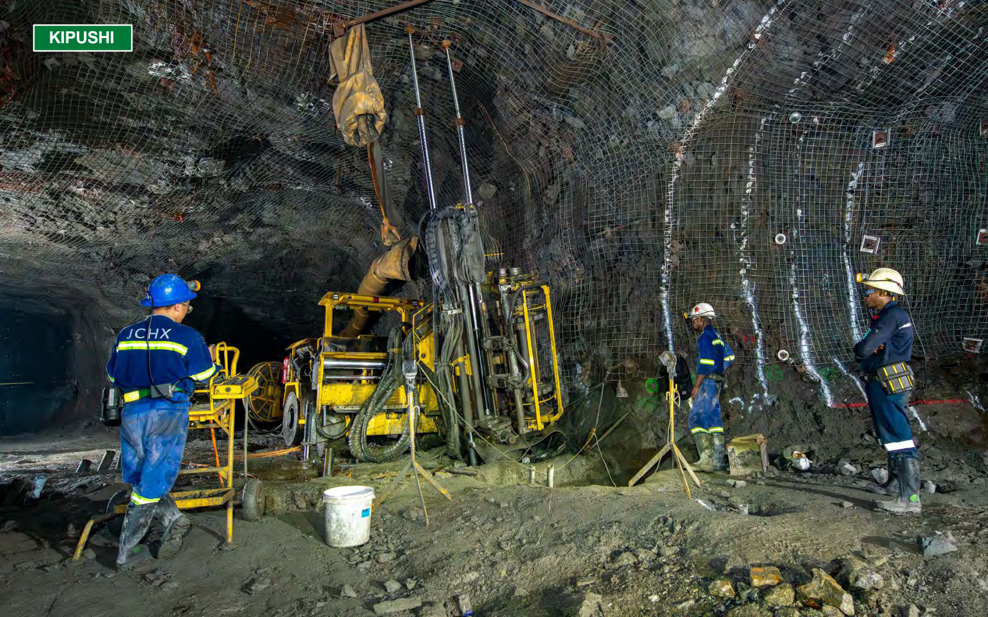
Simba long hole rig drilling the first slot raise holes at the 1,245 metre-level stope.
