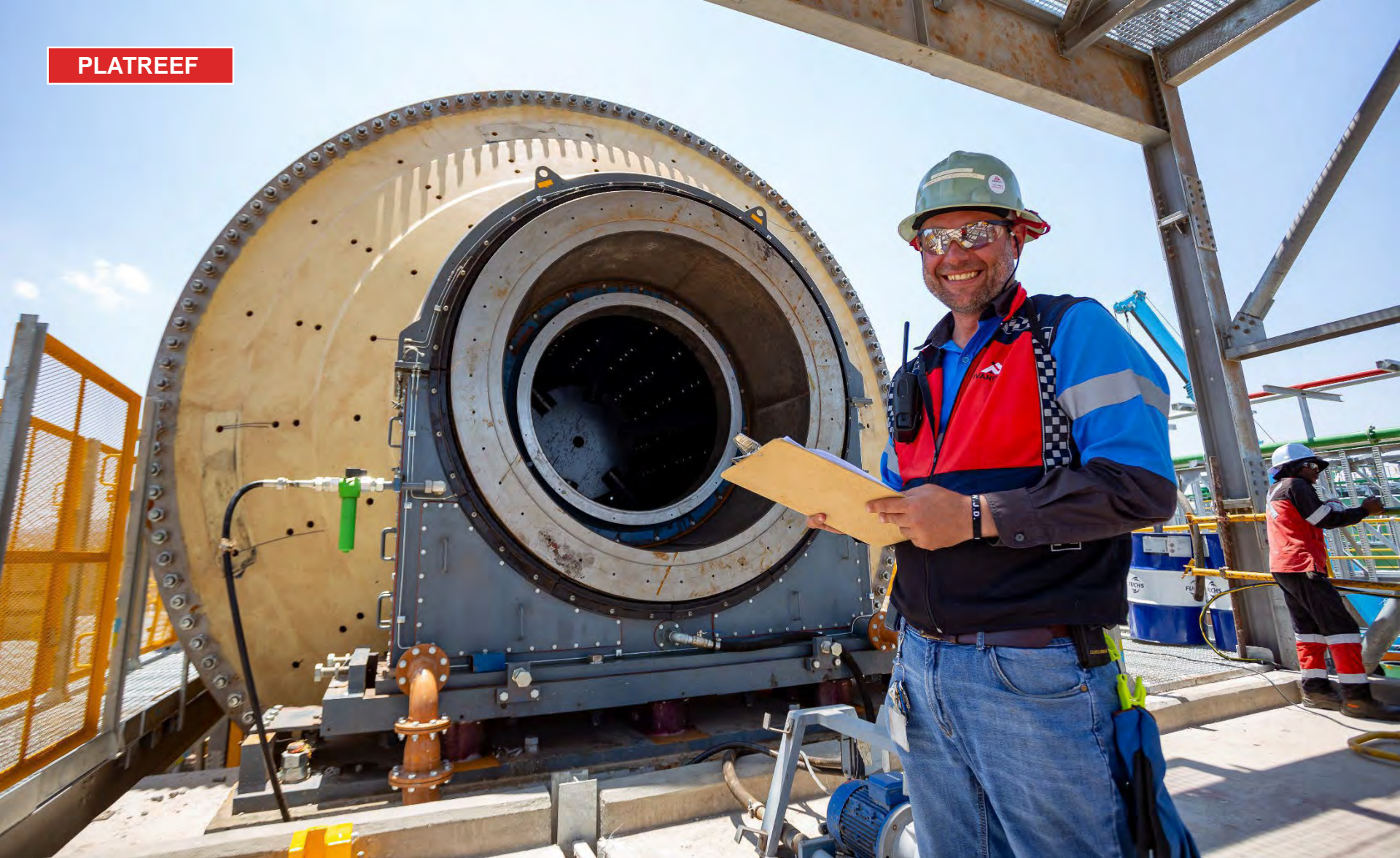
Jean-Pierre Fouche, supervisor, in front of the newly-installed Phase 1 ball mill, oversees construction activities at Platreef's concentrator site.
