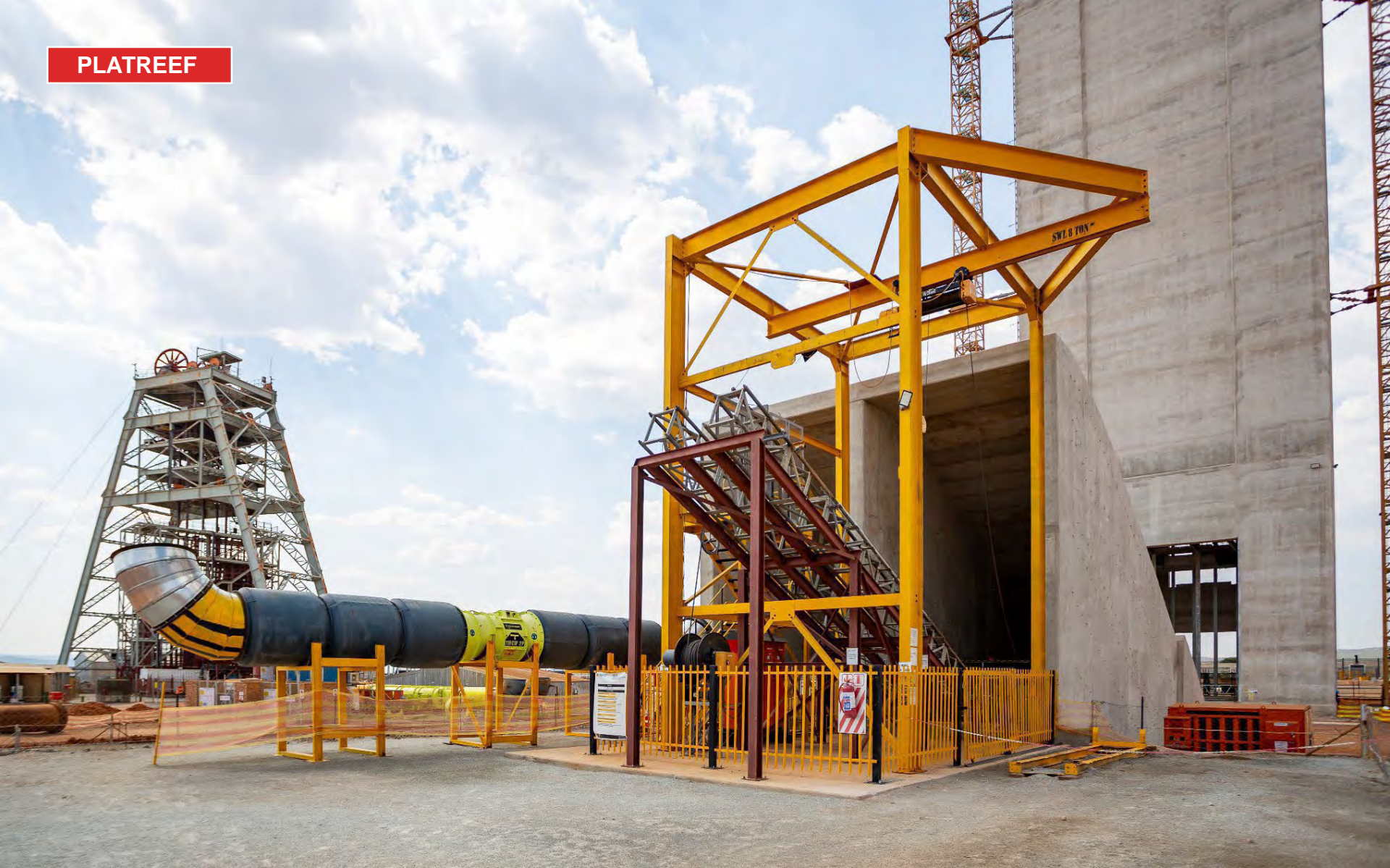
Platreef Shaft 2 ventilation plenum with Shaft 1 in the background.
