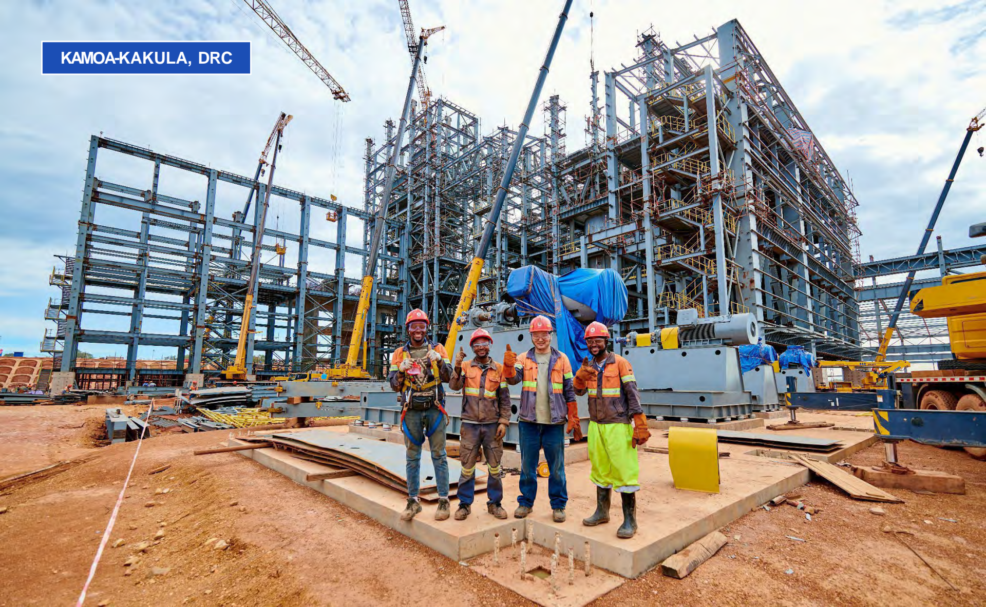
Construction crew in front of Kamoa-Kakula's Phase 3 direct-to-blister furnace. The smelter project is progressing on schedule for completion in Q4 2024.
