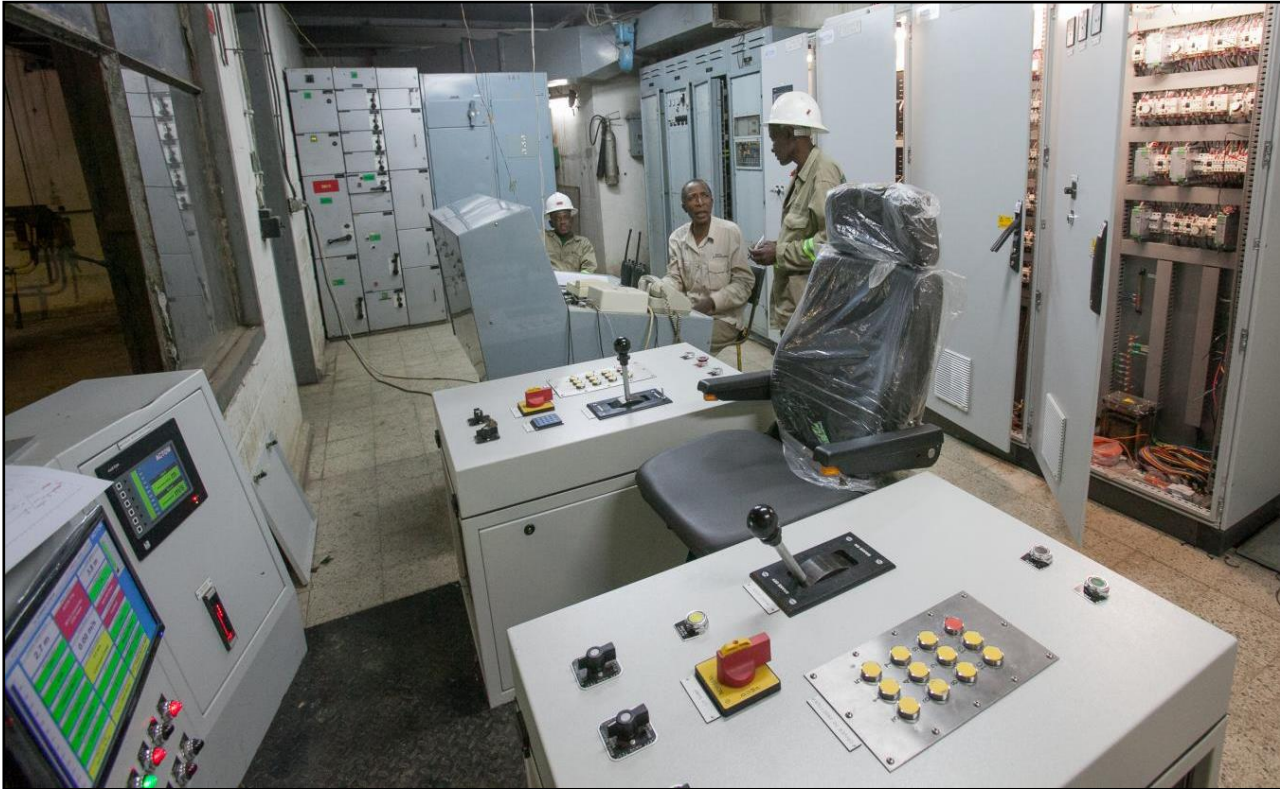
Figure 7: New winder control centre at Shaft 5.
