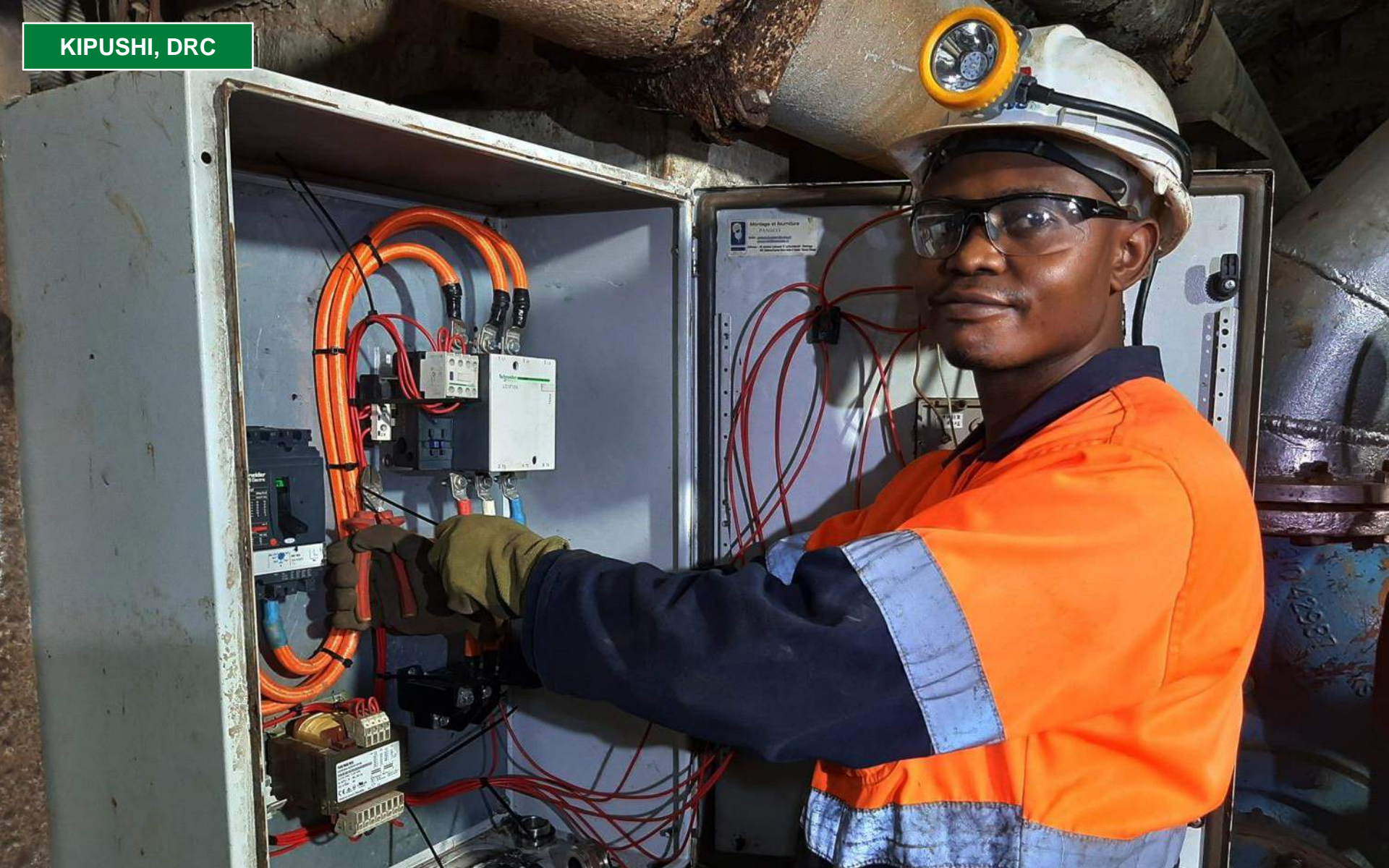
Espadon Ngambwa, electrician, installing an electrical panel for a new Flygt water pump at Kipushi's 700-metre-level.
