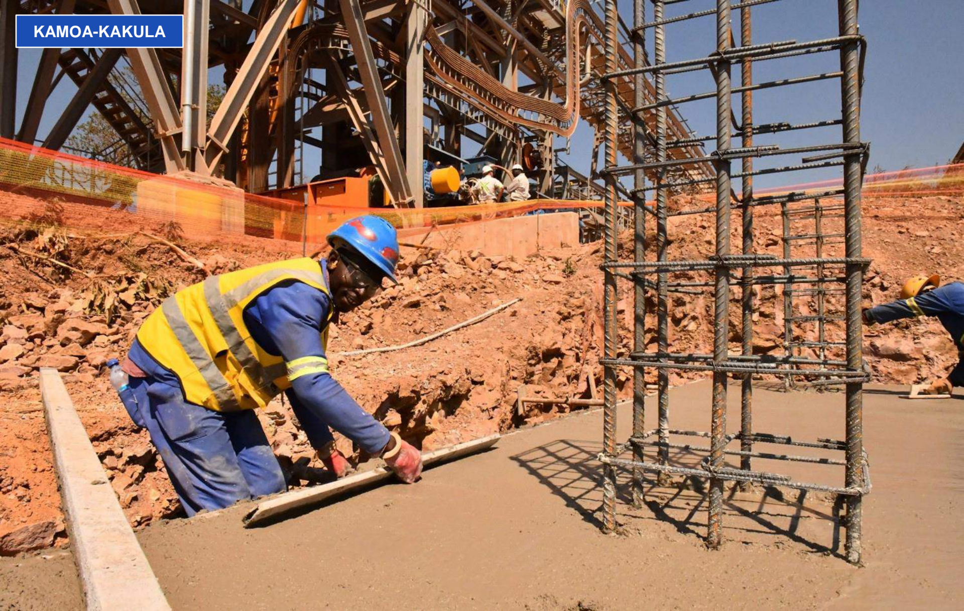
Mardoché Kilwa, a Kongo River employee, levelling a new concrete slab for a support structure for the conveyor belt extension.
