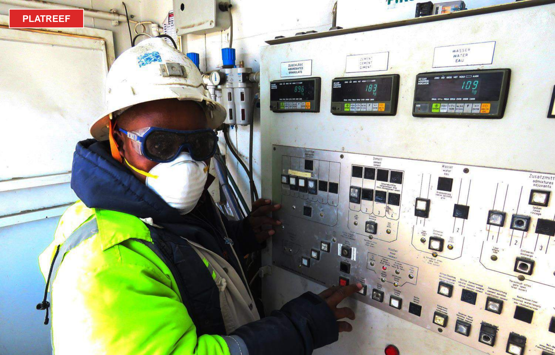
Ben Komape (Batch Plant Operator) at the control panel for Platreef's batch plant that makes concrete for use in the underground operations.
