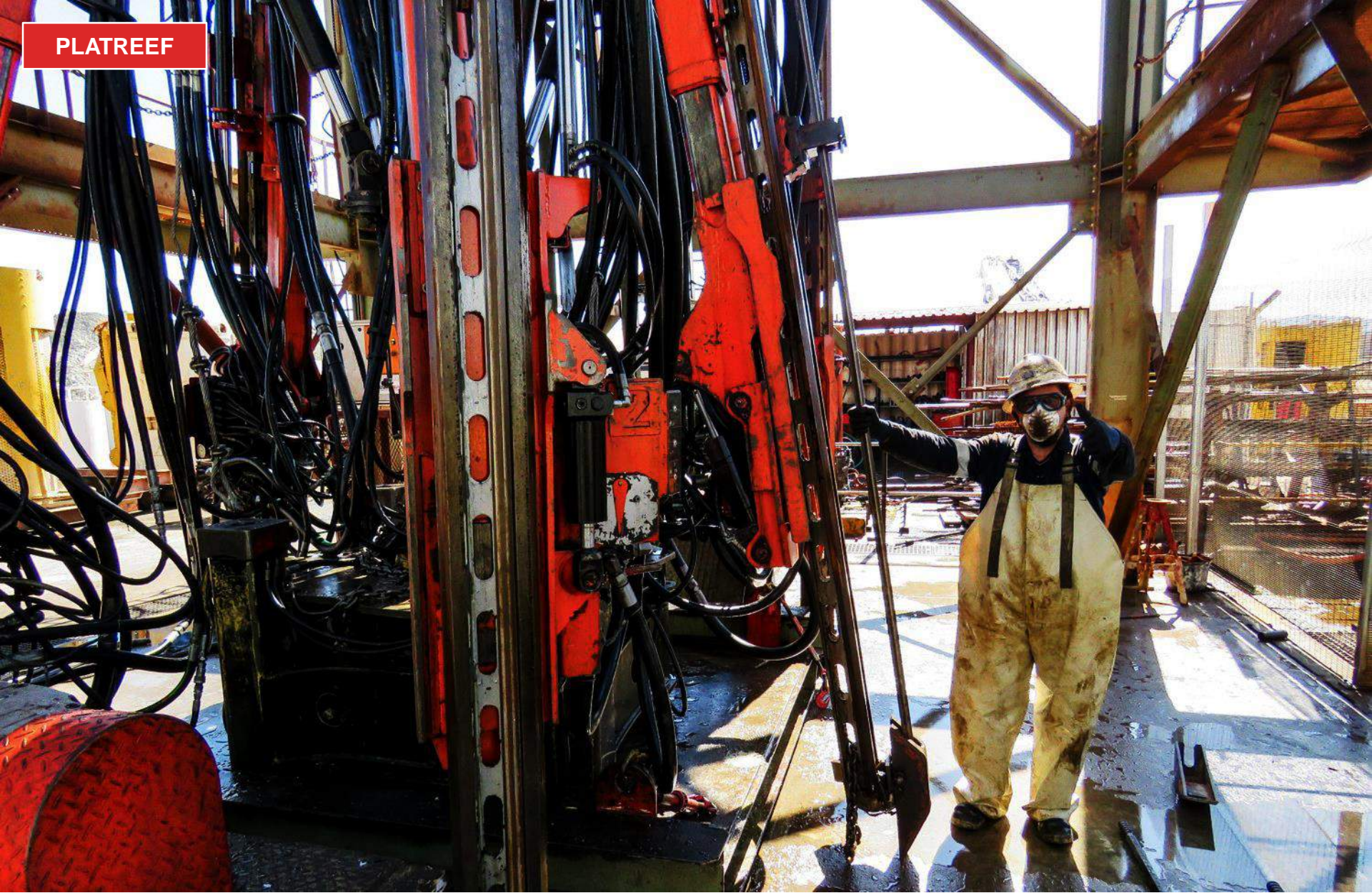
Dries Lombaard (Jumbo Fitter) performing routine maintenance on the six-boom jumbo drill used in shaft-sinking operations.
