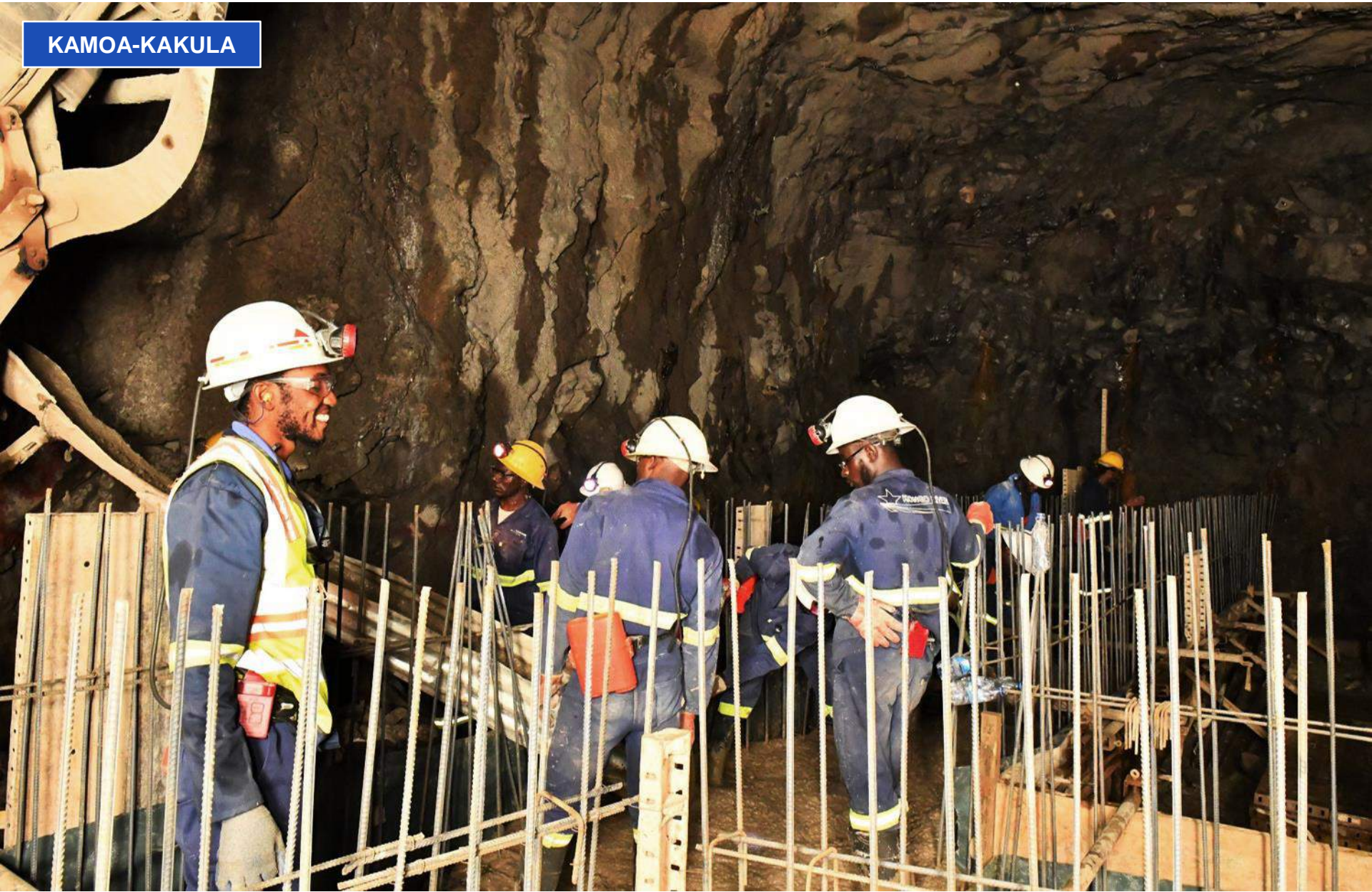
Members of DRC-based construction contractors, Kongo River, pouring concrete at electrical substation #3 in Kakula's southern decline.
