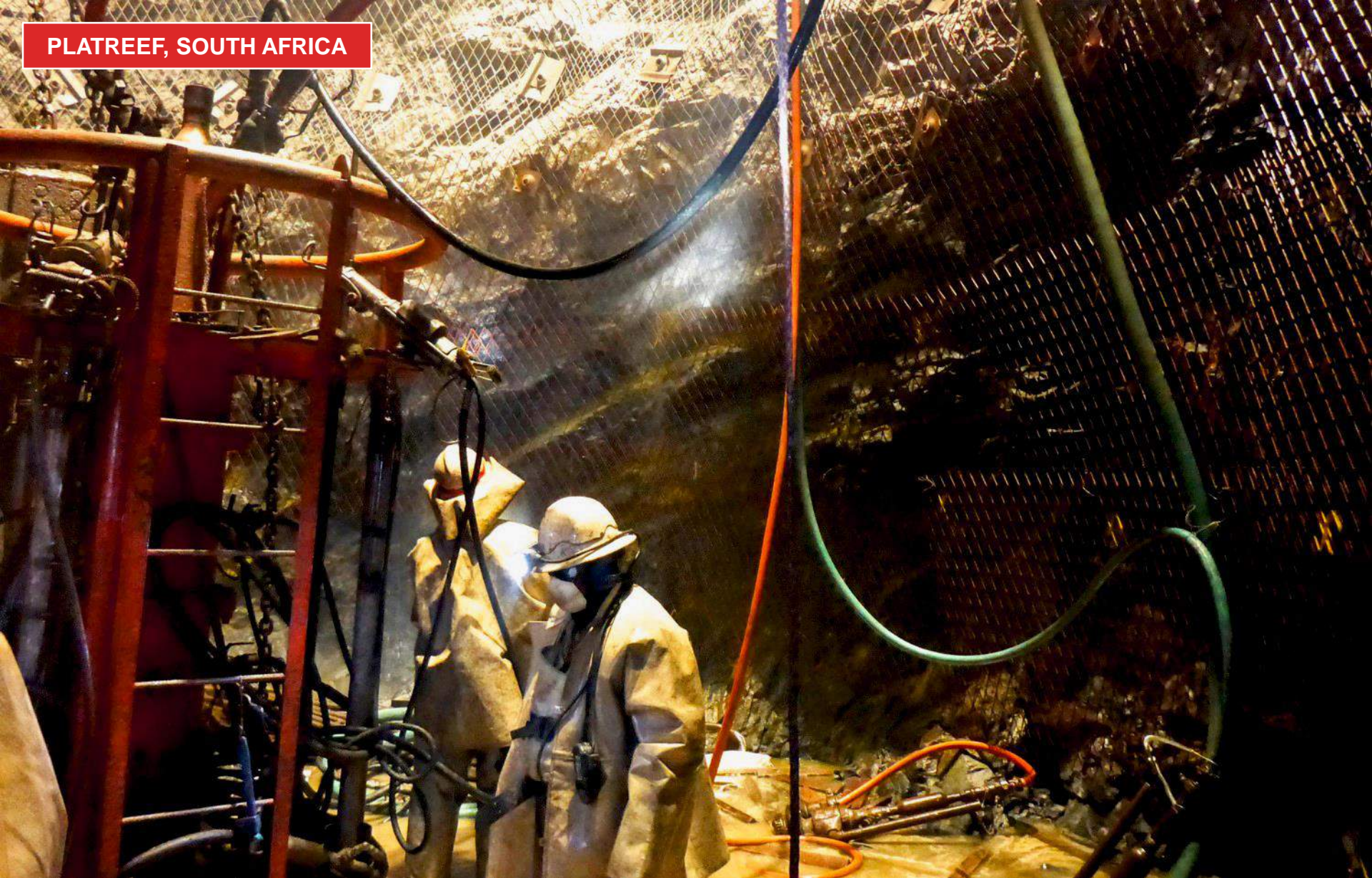
Shaft-sinking crew members installing side-wall support meshing in Shaft 1 at a depth of 982.6 metres below surface.
