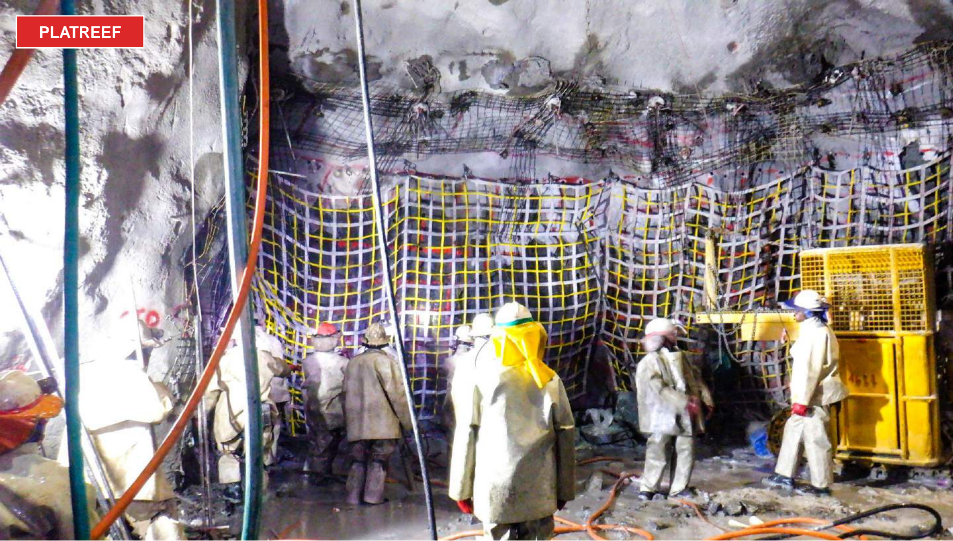
Rockdrill operators preparing to drill shotholes for the next development blast at the 950-metre-level station.
