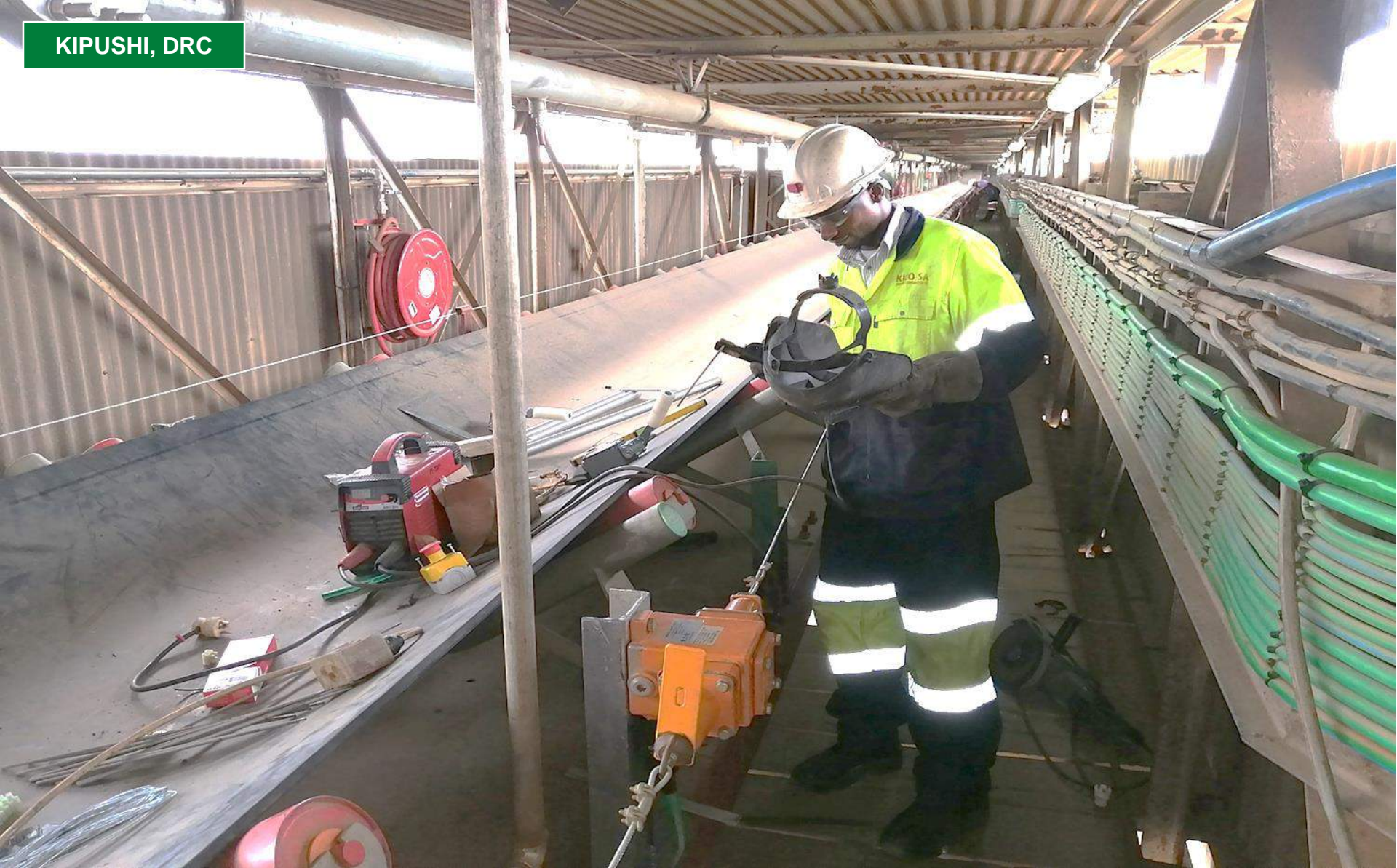
Kaboya Geullord installing brackets along Kipushi's T4 conveyor belt that will transport ore from the underground mine to surface.
