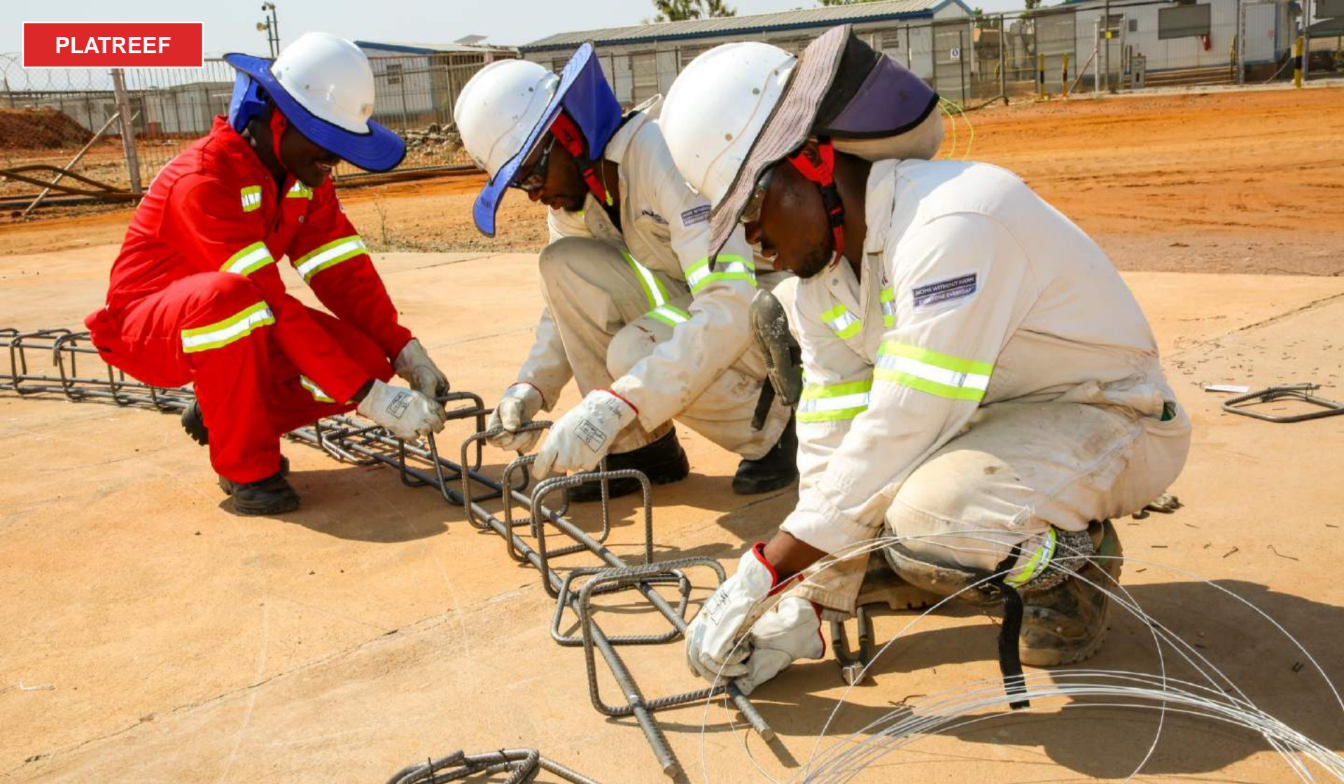
Amos Ledwaba (left), Tebogo Malope (centre) and Thabang Baloyi (right) preparing support steelwork for Shaft 1's 950-metre-level station.
