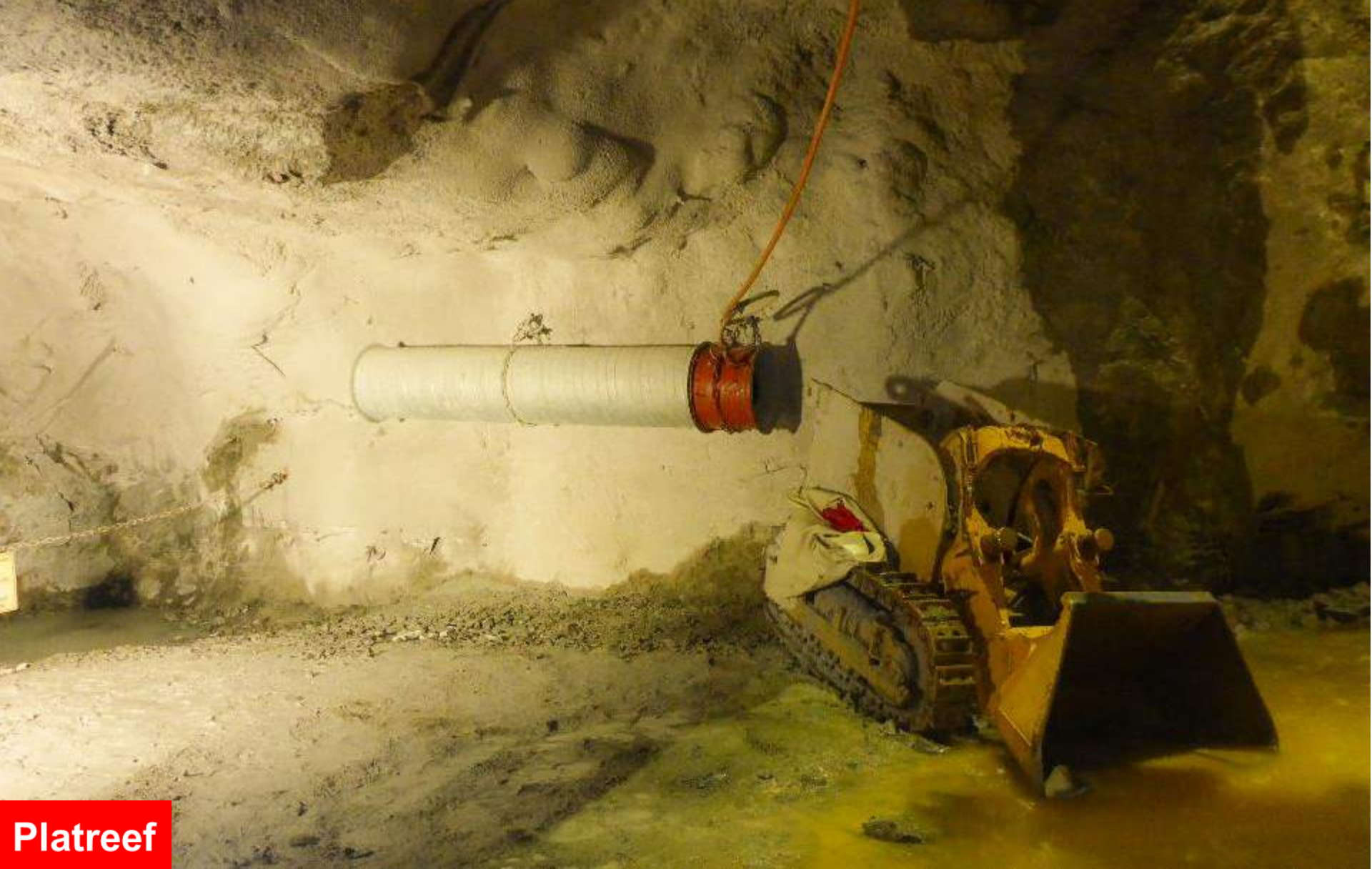
Underground mucking machine used to remove broken rock from the development of Shaft 1's 850-metre-level station.
