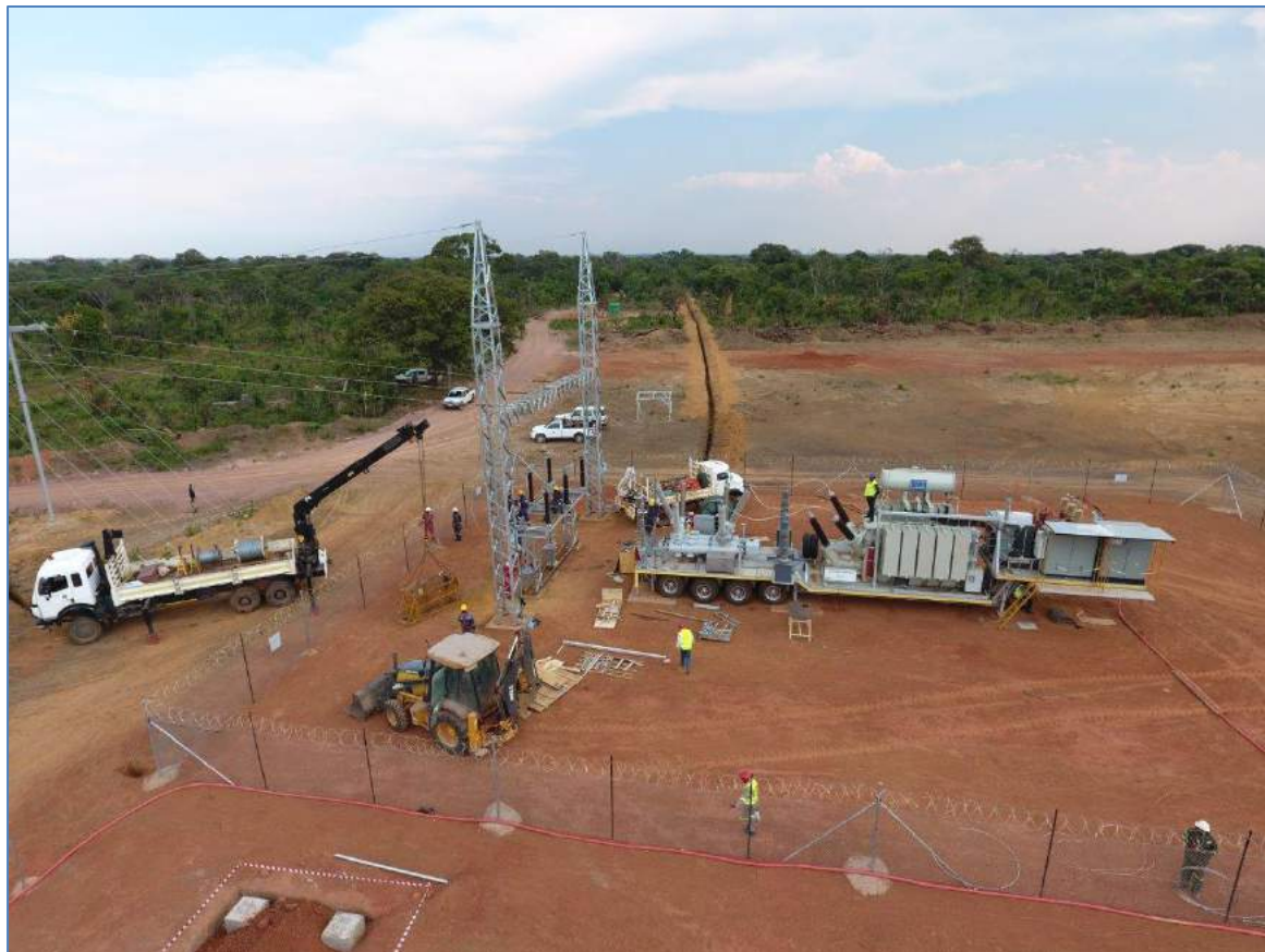
Figure 18.4 HV Mobile Substation Installed at Kansoko, October 2016
