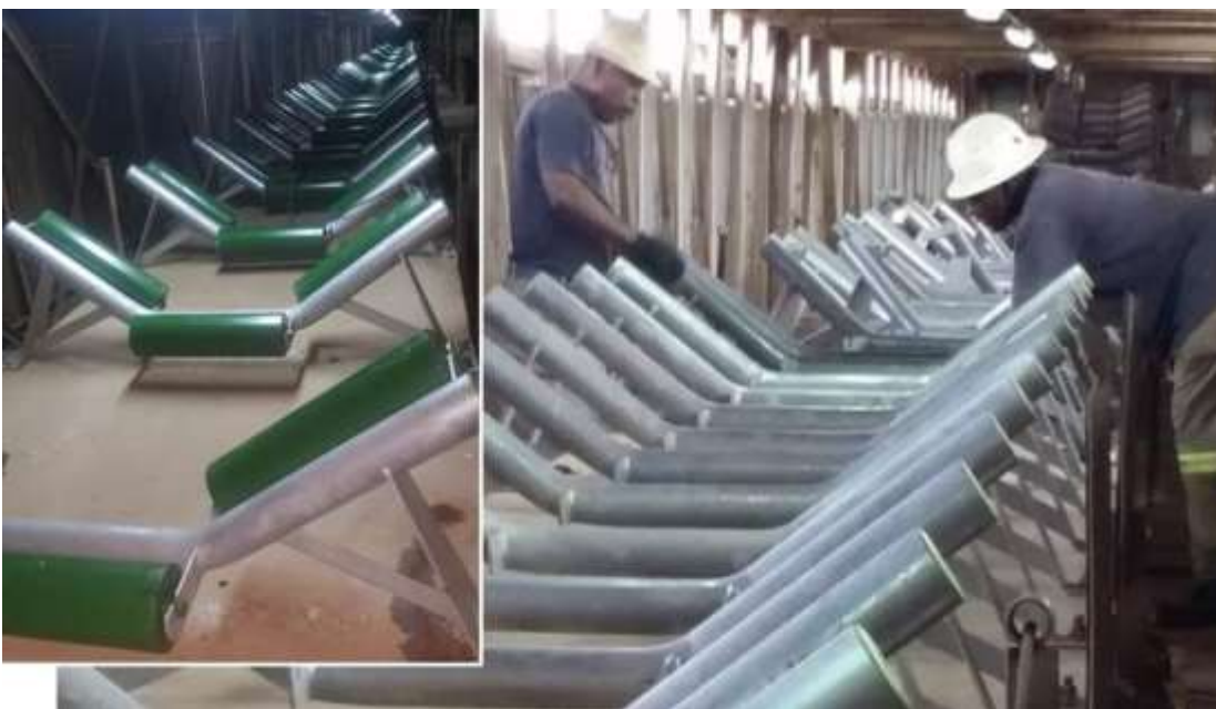
Figure 12: New idlers and rollers being installed on the ore conveyor belt as part of Kipushi's upgrading.
